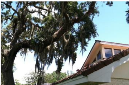
Tree Branches Hanging Over Roof
