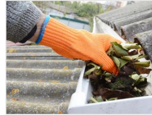
Debris in Gutter
