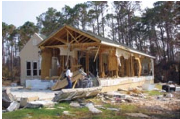
Flood water from Hurricane Ivan exceeded the required elevation of the top of the lowest floor supported by the stem wall foundation for this house leading to severe damage caused by waves and debris impact.
