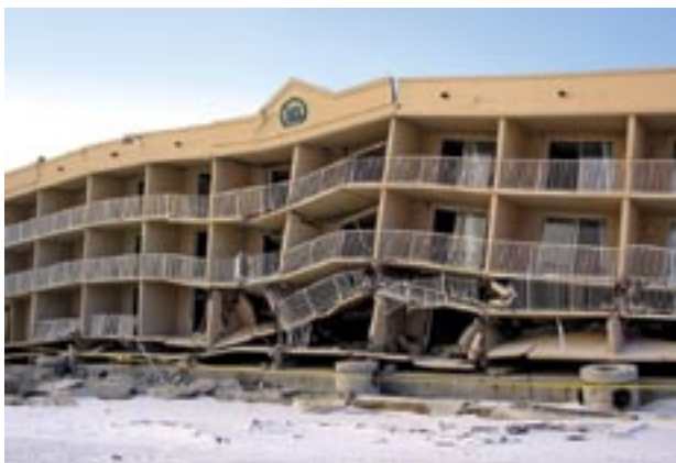
A multi-family condominium collapsed after Hurricane Ivan due to erosion of supporting soil under the shallow foundation.
