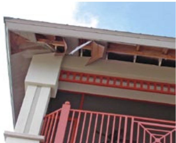
Soffit damage on the third story of a multi-family building. (Captiva Island)
