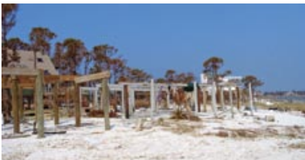
Several structures were completely torn off their pile foundations during Hurricane Ivan as a result of significant flood depths, waterborne debris impacts, and lack of connections.
