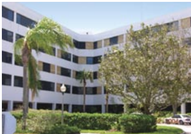
Aggregate from the Indian River Memorial Hospital's roof (Vero Beach) broke several of the patient room windows (which were covered with plywood after Hurricane Frances).
