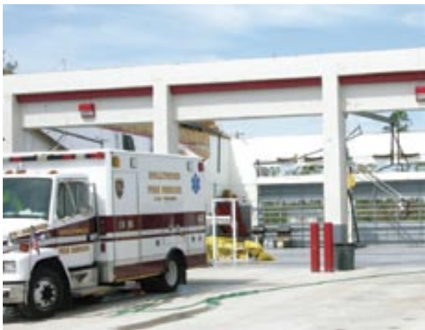
Failure of three of six new doors on a fire station in Charlotte County resulted in the loss of the entire roof structure over the apparatus bay during Hurricane Charley.
