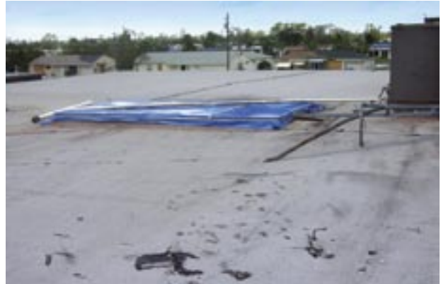
A large HVAC package unit was blown off this curb during Hurricane Charley. Note the loose LPS conductors this side of the curb. This school had significant damage from several pieces of rooftop equipment that blew off the building roof. (Port Charlotte Middle School)
