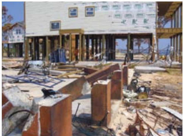
High flood levels during Hurricane Ivan and lack of structural capacity to withstand waves and debris loads caused this reinforced pier foundation to fail.
