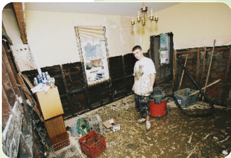
A Bridgeville, Pennsylvania, resident cleans up after a flash flood caused by two tropical storms that struck the area within a two week period in September 2004. All the baseboards and insulation had to be removed to prevent an outbreak of mold and mildew. Bob McMillan/FEMA
