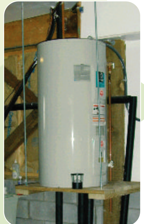
This water heater in the basement of a home has been elevated to protect it from flood. Dave Saville/FEMA
