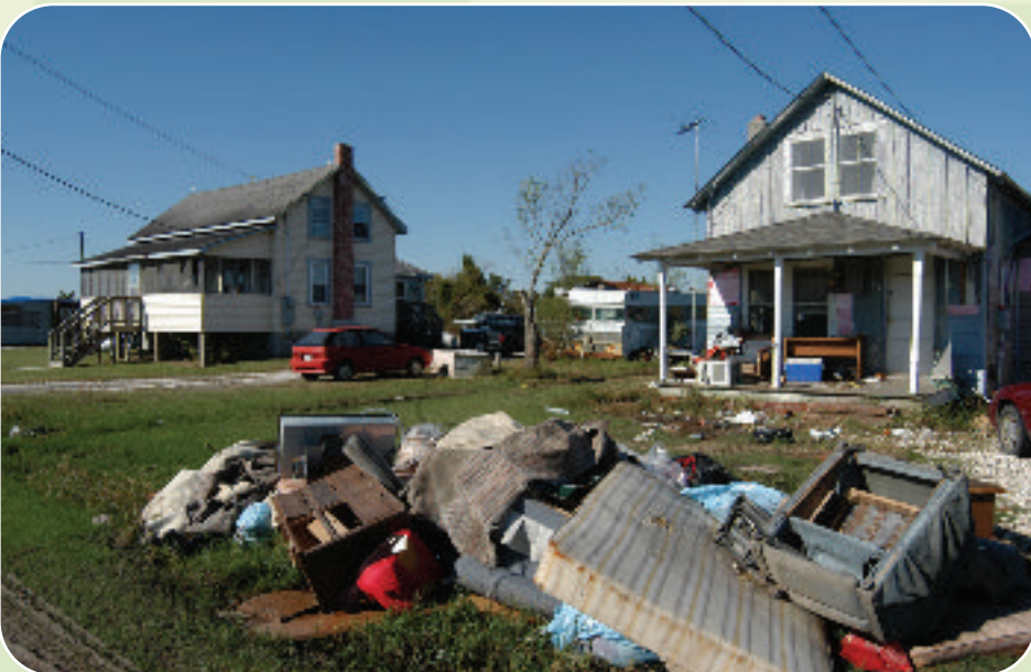
Two houses side by side in Englehard, North Carolina. The house on the right was not elevated and suffered flooding in October 2003 due to Hurricane Isabel. While the house on the left experienced the same storm, it was not flooded because it had been elevated with FEMA mitigation funds. Mark Wolfe/FEMA
