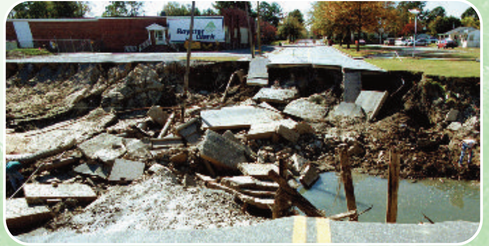
Floodwaters across this road in Tarboro, North Carolina, hid a dangerous road washout. Dave Gatley/FEMA
