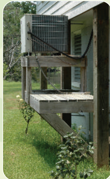
When elevating a structure to mitigate against flooding, it is important to elevate outdoor appliances as well, like this air conditioning unit. Mark Wolfe/FEMA
