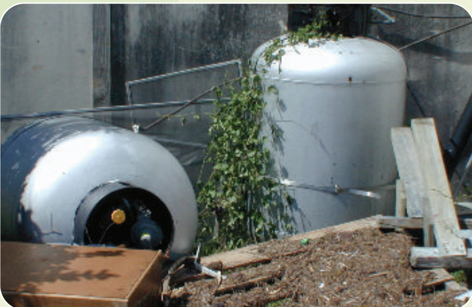
Straps held these fuel tanks in place during a flood. Dave Gatlley/FEMA
