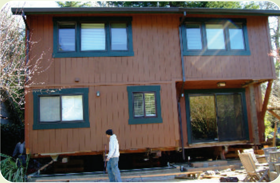
A Marin County, California, resident raises his home to avoid further repetitive losses caused by flooding from a nearby creek. Adam Dubrowa/FEMA
